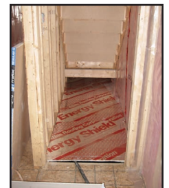
A blocked stairway traps CO from a heater that is running in the basement
