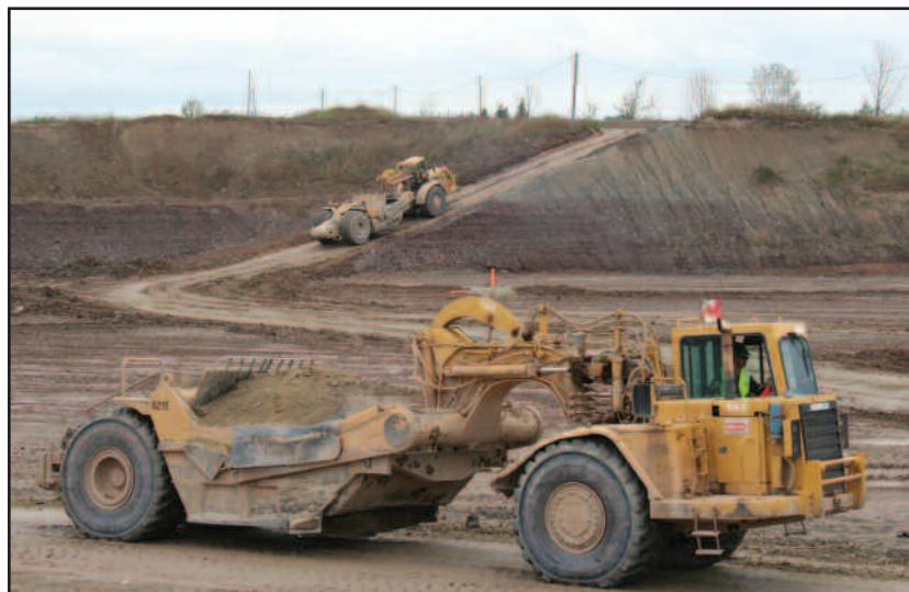
Organize the site so vehicles can drive through and don't need to back up.
